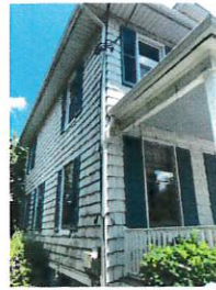
VIEW FROM FRONT LOOKING AT WEST SIDE OF HOUSE WHERE ADDITION IS LOCATED
