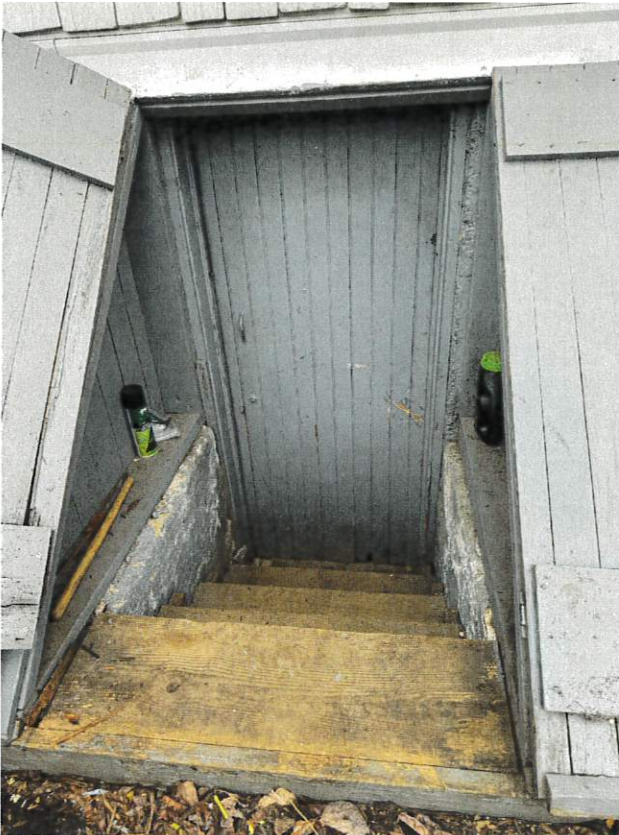
Photo of current basement egress door that may be replaced to code:
