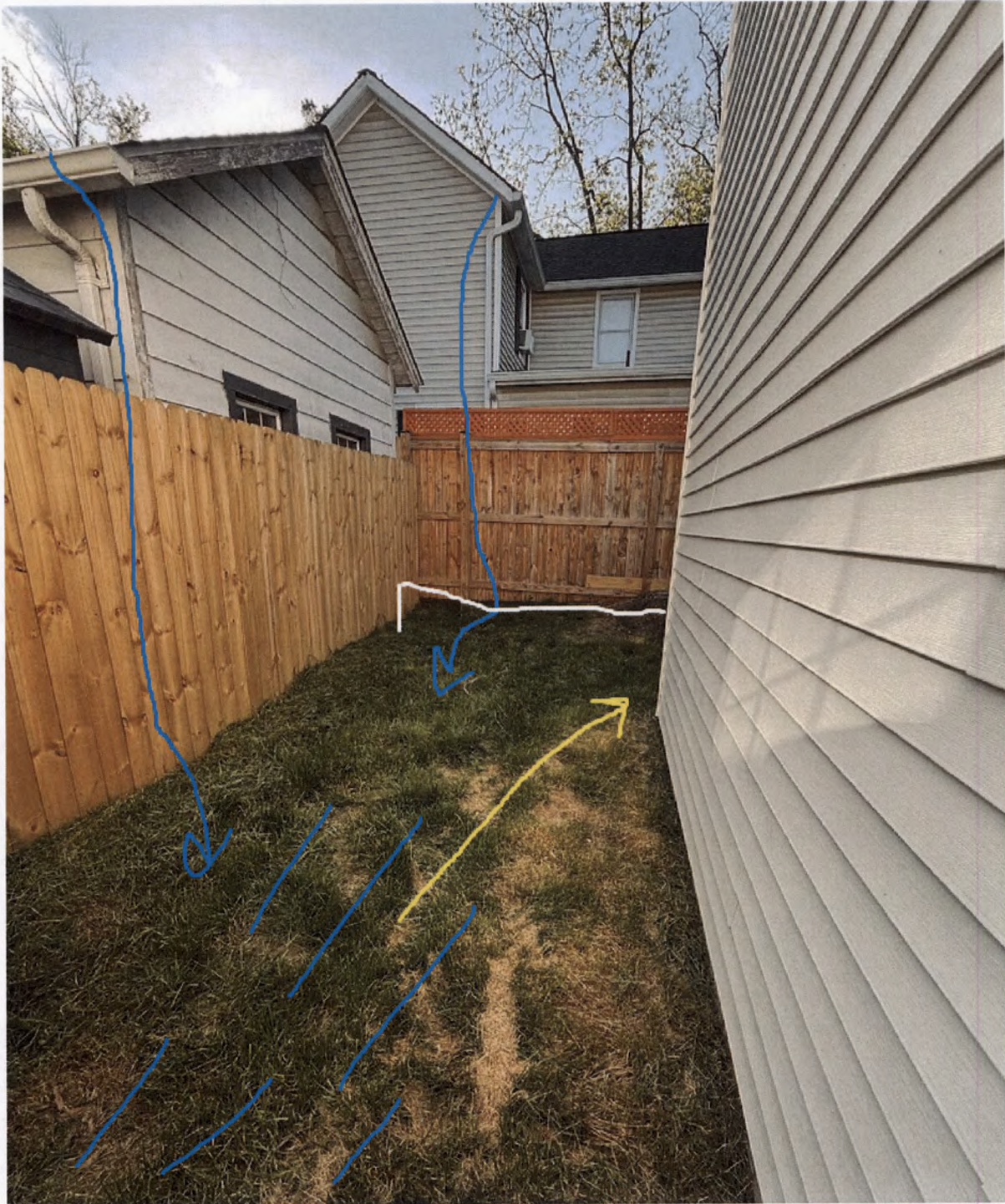
Figure 3: Annotated of stormwater runoff from nearby downspouts (Blue Arrows) to where the water stagnation issues are (Blue Stripes) and where the overflow drain will be trenched out of the corner downslope (Yellow).
