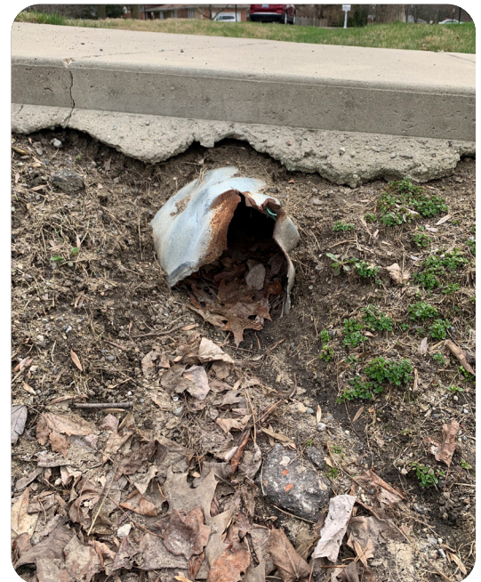
Damaged storm sewer culvert (Giffels Webster)
