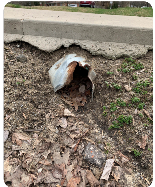
Damaged storm sewer culvert (Giffels Webster, 2020)
