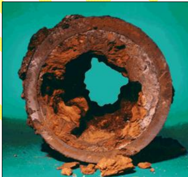
Image 1 – Pipe with Severe Tuberculation
