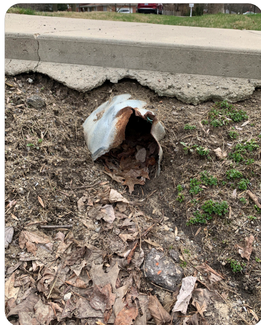
Damaged storm sewer culvert (Giffels Webster, 2020)
