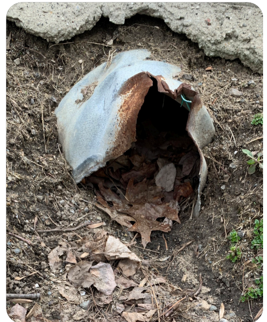
Damaged storm sewer culvert (Giffels Webster)
