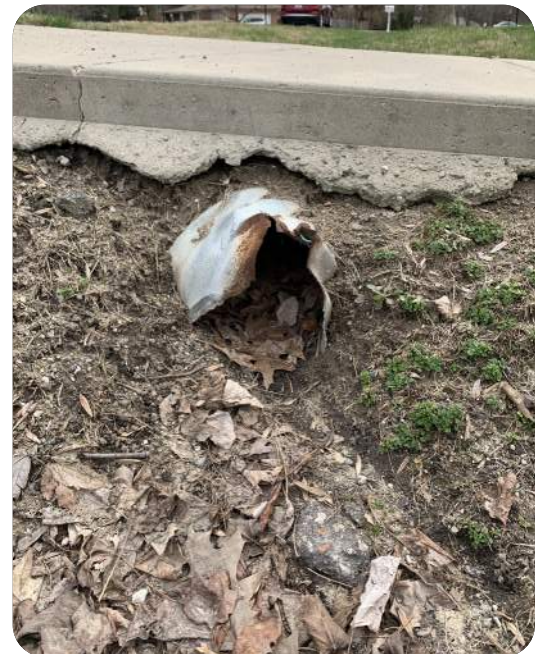
Damaged storm sewer culvert (Giffels Webster, 2020)
