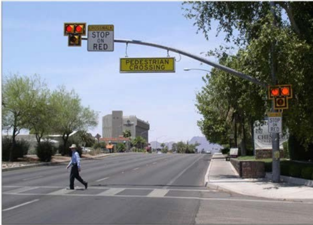
HAWK signal in Tucson, AZ. Source: Federal Highway Administration (FHWA)
