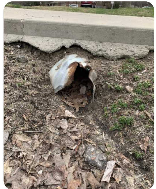
Damaged storm sewer culvert (Giffels Webster, 2020)
