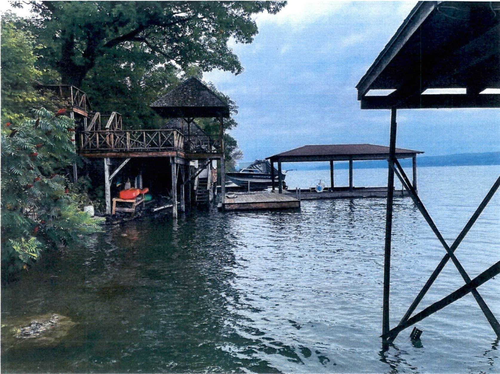
View of Lakeshore Structure at 295 Bill George Rd from boardwalk of 281 Bill George Rd. on Friday, Aug 27th, 2021.
