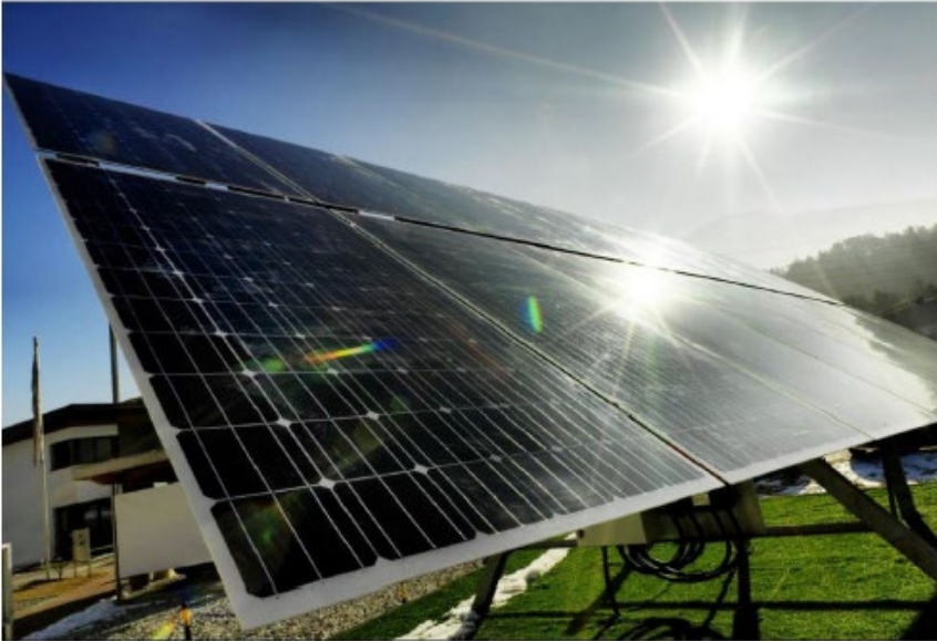
Solar panel showing solar glare
