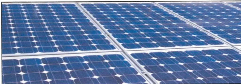
Figure 11. Module Spacing Gaps
