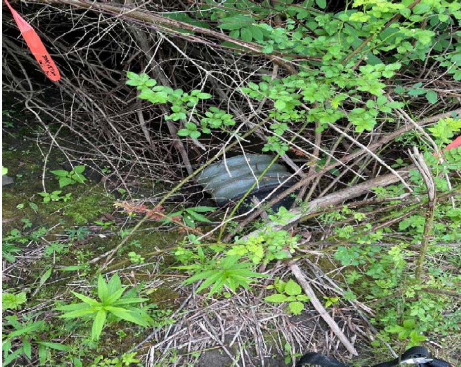
Photo 13. View looking at a pipe culvert feeding water from the northern arm of the 'E' flagged wetland towards the 'E' flagged wetland to the south.
