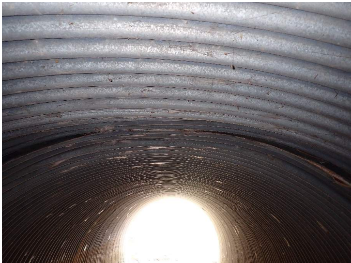
VISIBLE DEFLECTION IN CEILING AT WEST SEAM
