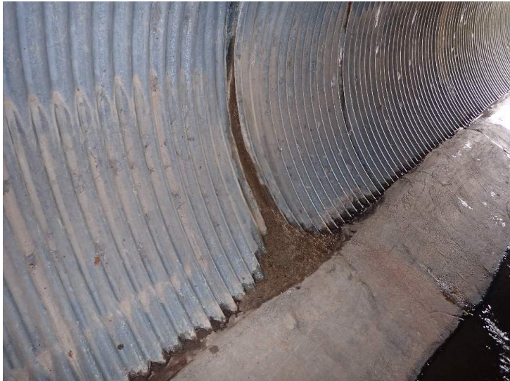
WEST SEAM, NORTH SIDE OPEN WITH MINOR INFILTRATION
