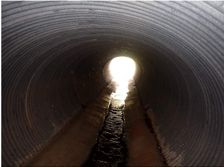
MIDDLE OF CMP VISIBLY SQUASHING COMPARED TO END SECTION
