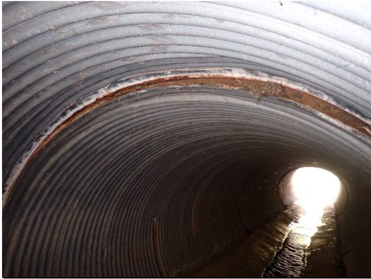
EAST SEAM OPEN 1.25IN, VISIBLE FILL
