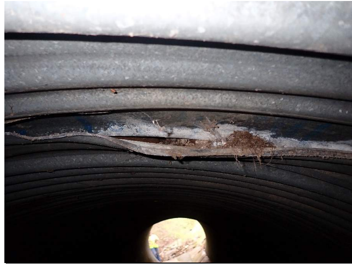
FILL VISIBLE AT TOP OF MIDDLE SEAM
