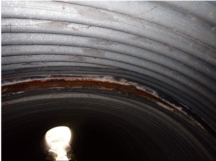
EAST SEAM OPEN 1.25IN, VISIBLE FILL
