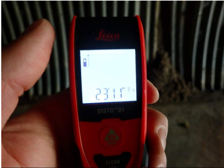
WEST SEAM LOC. 24FT FROM WEST INLET, NOT UNDER RDWAY
