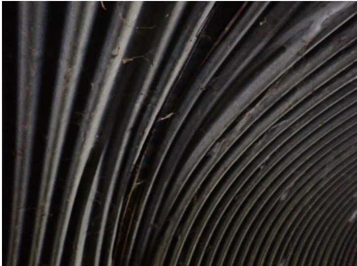
DIFFERENTIAL SETTLEMENT IN MIDDLE SEAM, NORTH SIDE
