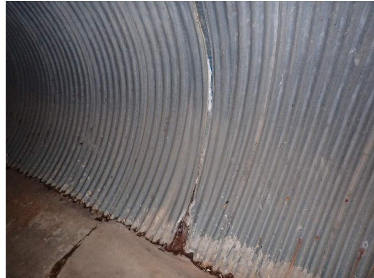
MIDDLE SEAM WITH MINOR LEAKAGE, NORTH SIDE
