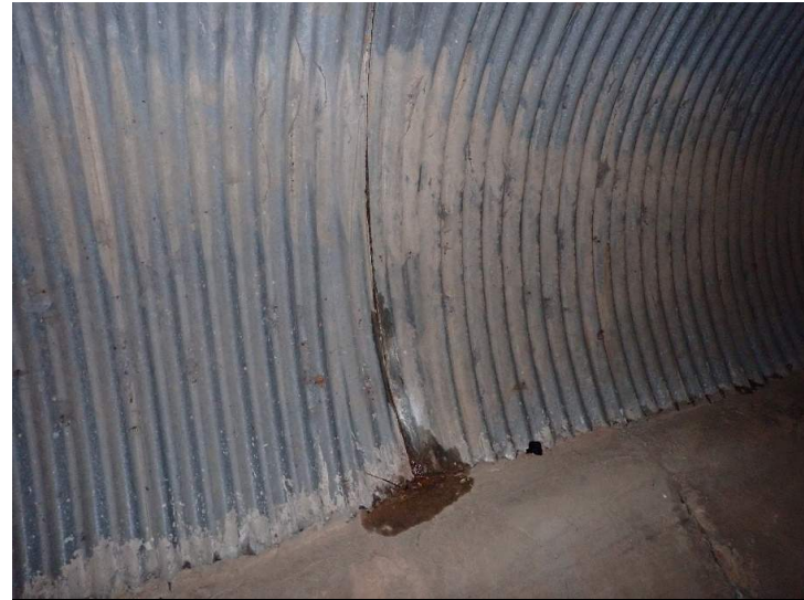
MIDDLE SEAM WITH MINOR LEAKAGE, SOUTH SIDE
