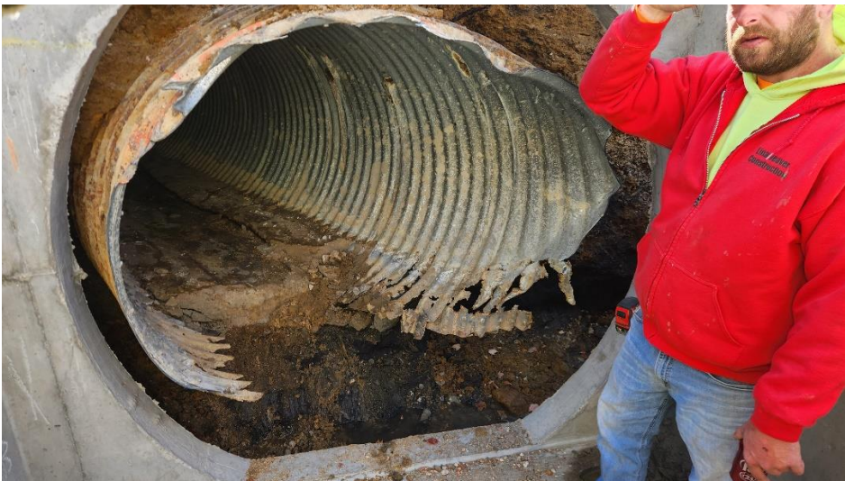
Photo #3 – Deterioration of existing 54" CMP at Junction Box JB-A2
