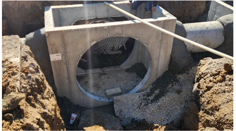
Photo #4 – Junction Box JB-A2 (looking south)
