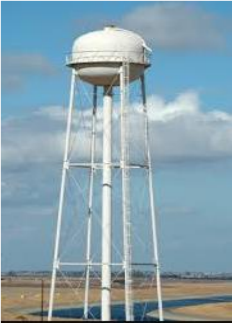
MULTI-LEG 100,000 GALLON WATER TANK
