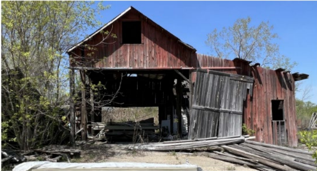
PHOTO 16-1 Barn and Lean-to - Poor Condition
