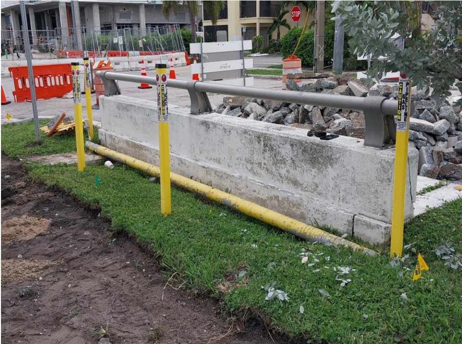
Photo of existing Lake Shore Drive bridge structure and adjacent gas line to be relocated
