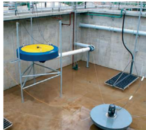
Emptied Alfa Laval AS-H SBR Reactor
