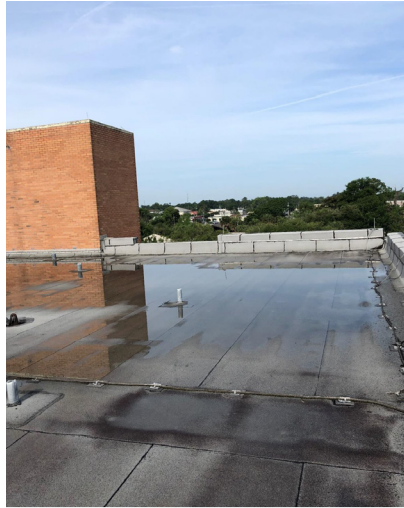
Standing water on roof
