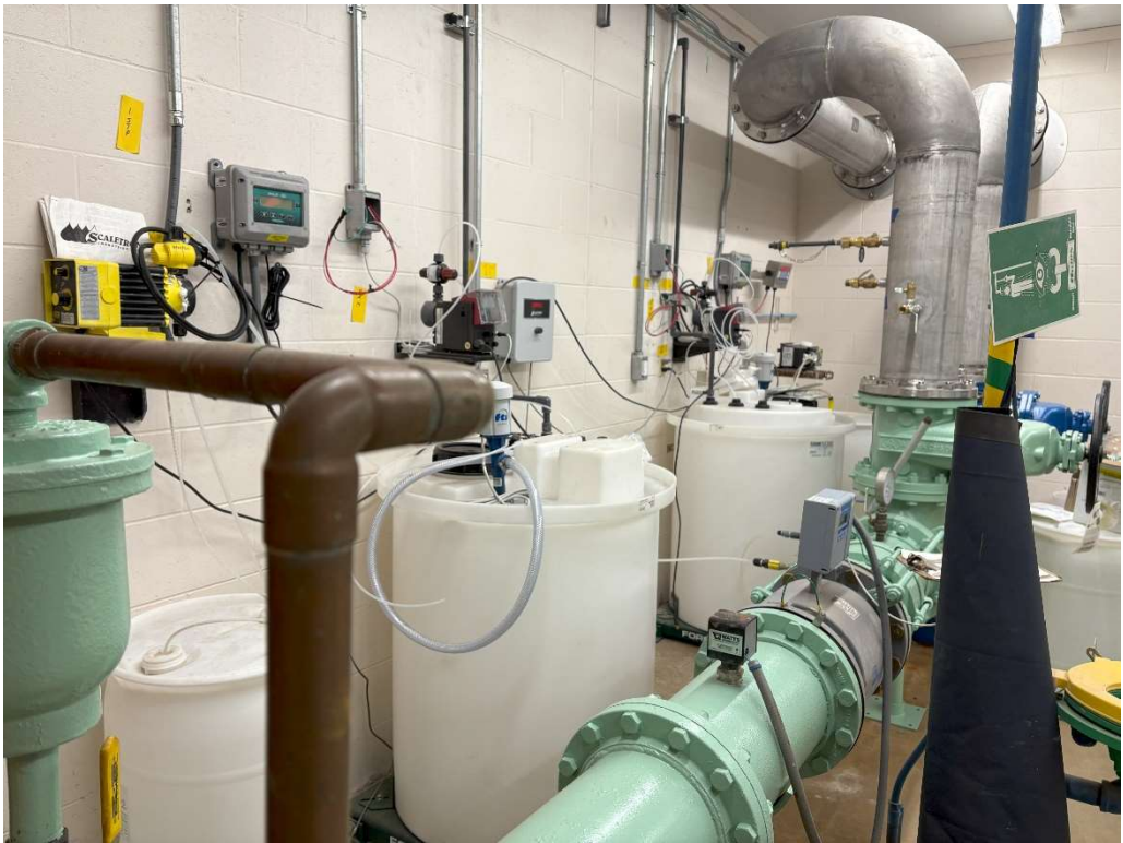
Chemical Feed Equipment Installed
