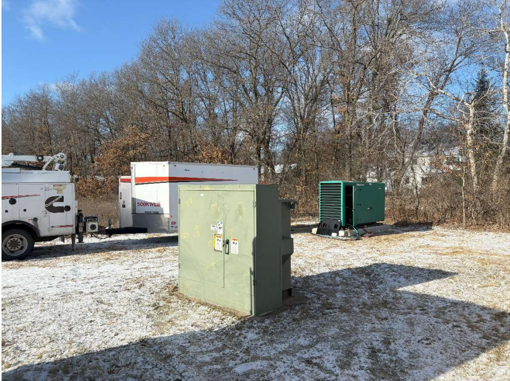
Generator Load Bank Testing
