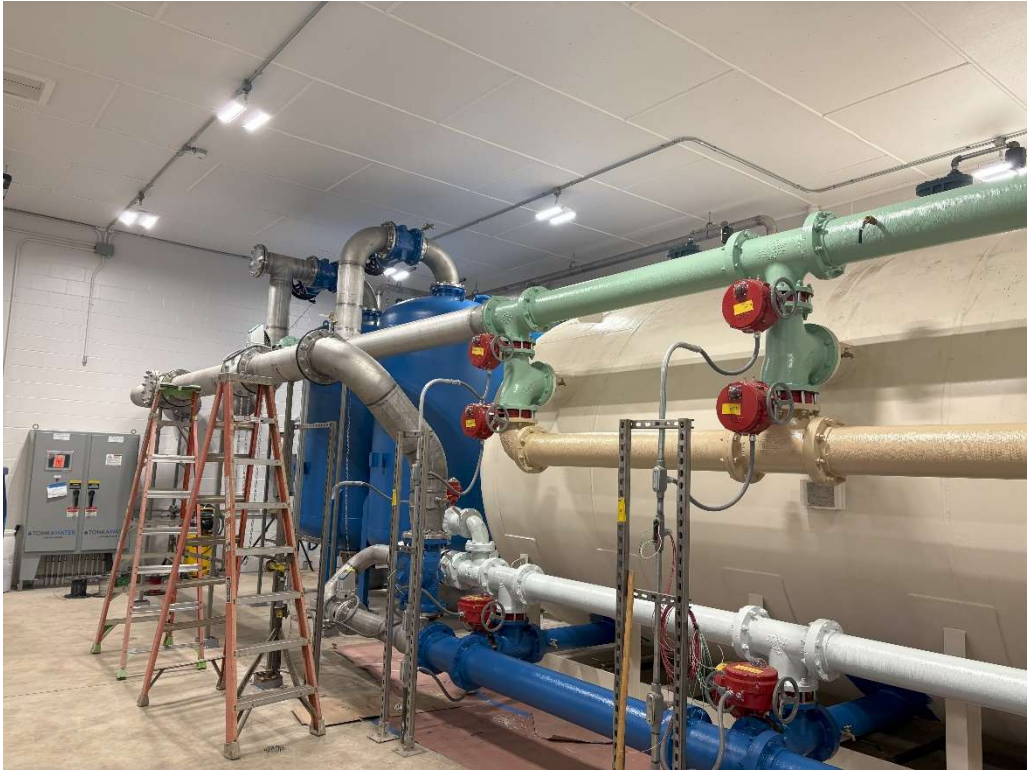
Coatings on Vessels and Piping
