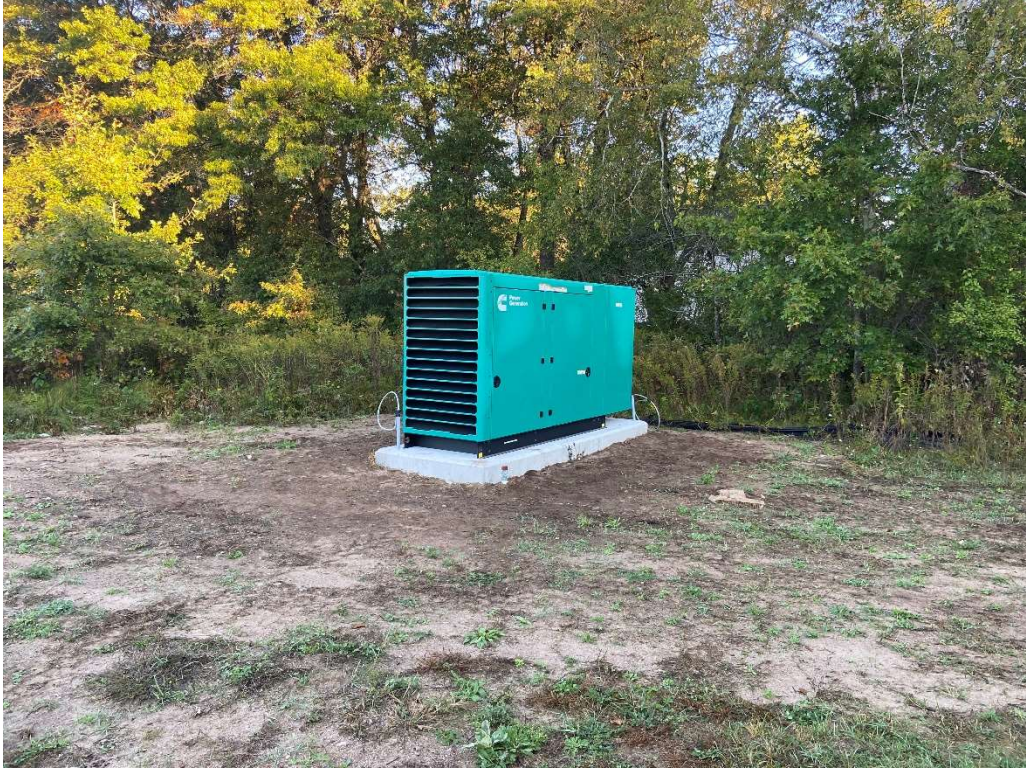
Generator Installed on Pad.
