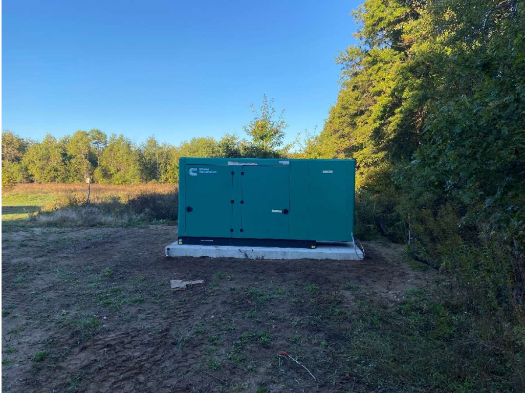
Generator Installed on Pad.
