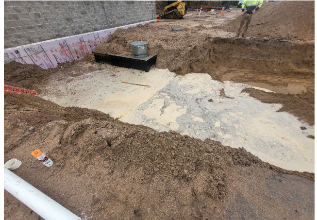
Water Filled Excavation Hole after WM Break
