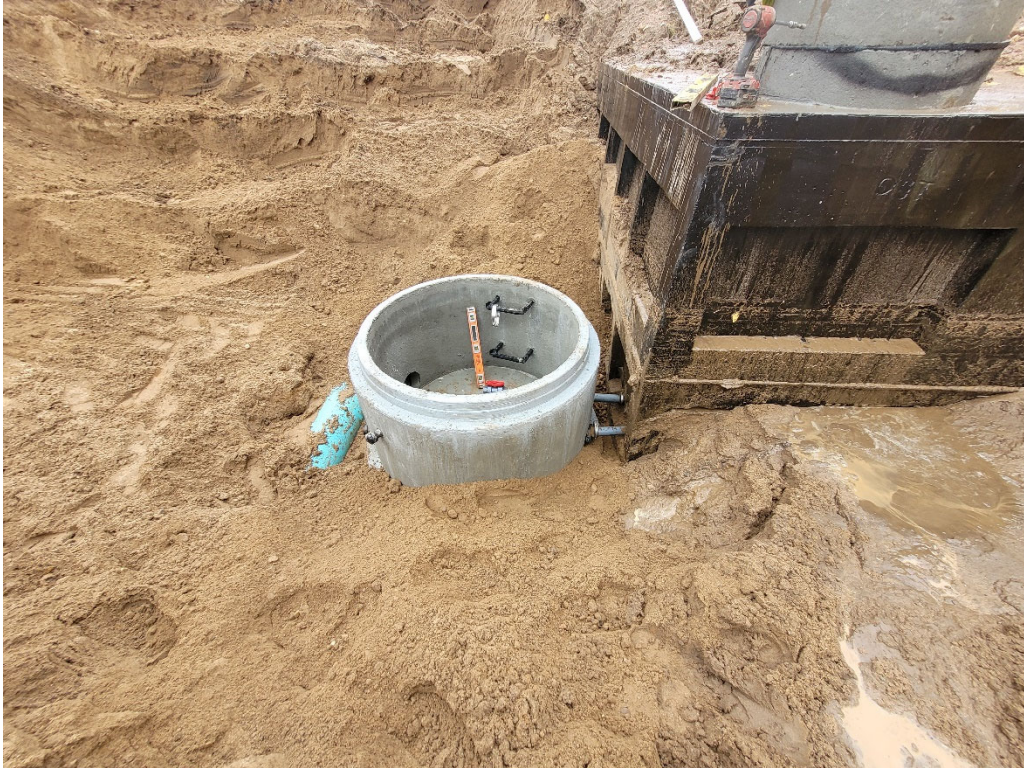
Underground backwash tank discharge manhole
