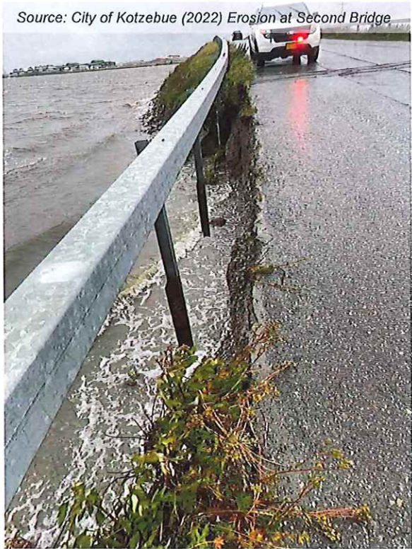
Figure 15: Erosion at Second Bridge (Kotzebue Slough)
