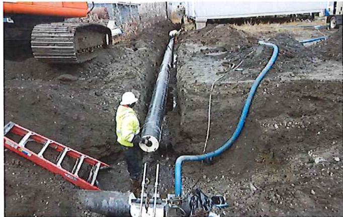
The DOWL team worked with the City in 2019 to replace a portion of Swan Lake Loop on time.
