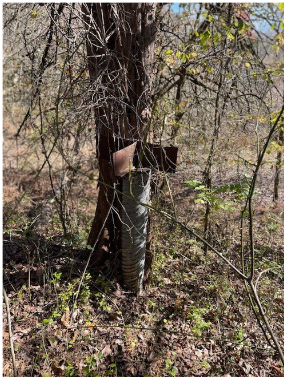
Old spillway pipe from failed pond construction WL-1
