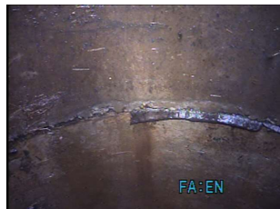
Manhole Defect Photos:
