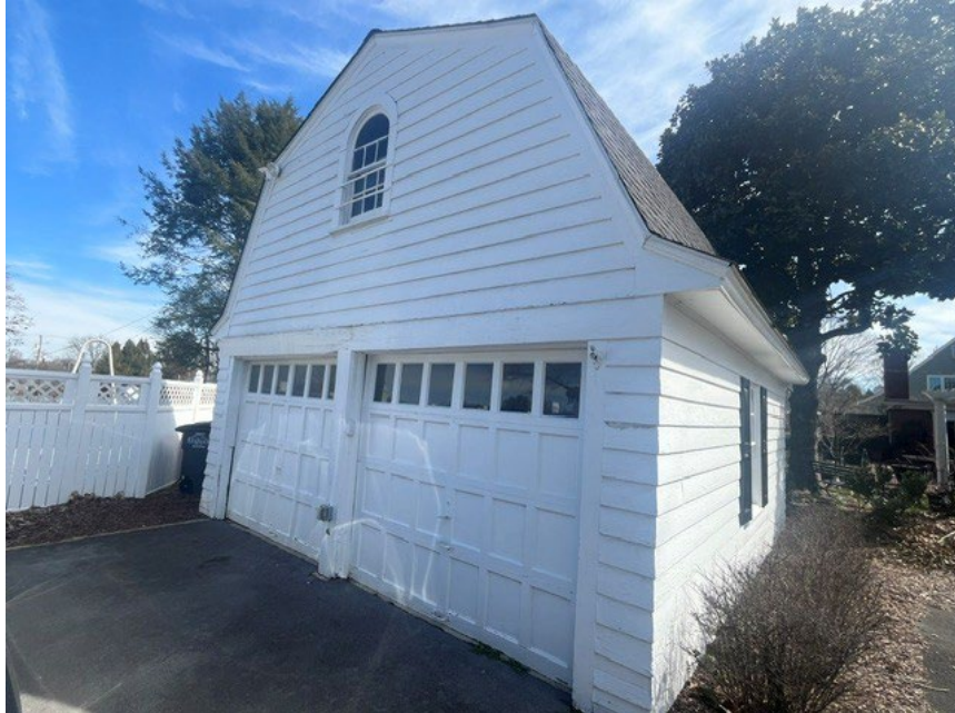
The existing garage will be restored, with an addition extending on the west side toward the pool area.
