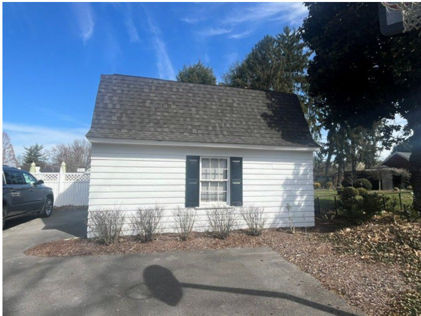
Side view of the existing garage facing the road—no changes planned for this side facing Watauga, except for window replacements.
