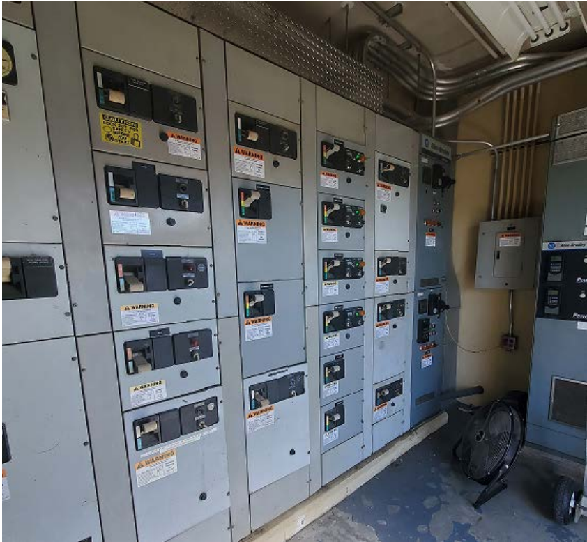
Motor Control Center (MCC) 6 – Installed in 1980 and single point of failure for critical process
