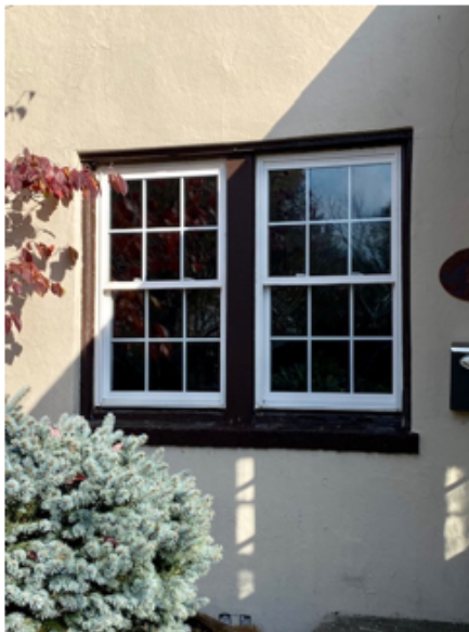
Picture of bottom left windows in living room area that were replaced. Old windows were rotten, had broken panes and were causing water damage to interior walls, baseboards and floors. Sorry, because of all the damage, I did not know I needed approval.
