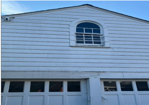
Areas of the garage exhibiting wear, aging, and potential concerns
