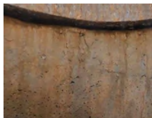
Manhole Defect Photos:
