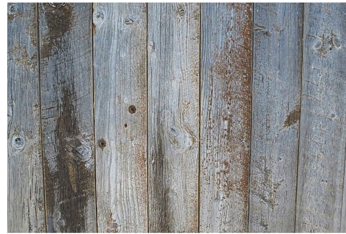
EXTERIOR FINISH 3 (EF-3): WOOD BOARD RAINSCREEN, VERTICAL MONTANA TIMBER PRODUCTS CORRAL BOARD
