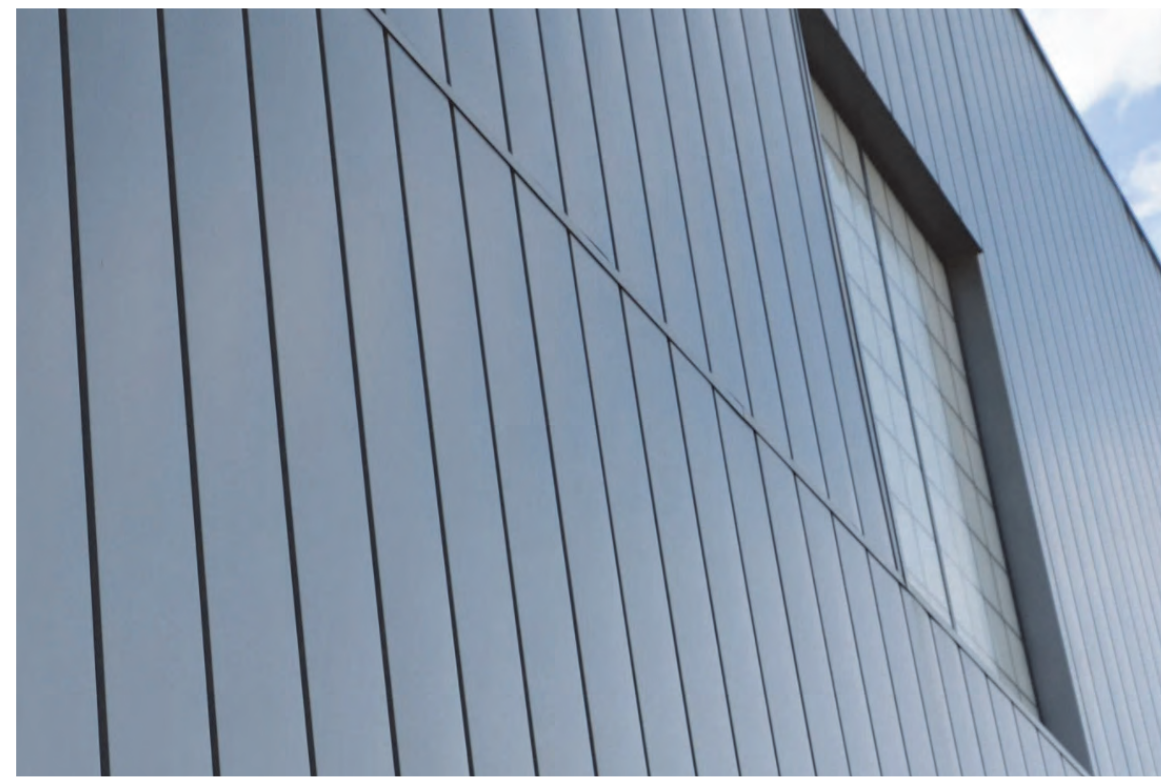
EXTERIOR FINISH 6 (EF-6): 12" WIDE METAL FLAT PANEL, VERTICAL SIDING, WESTERN STATES METAL ROOFING, MATTE PATINA
