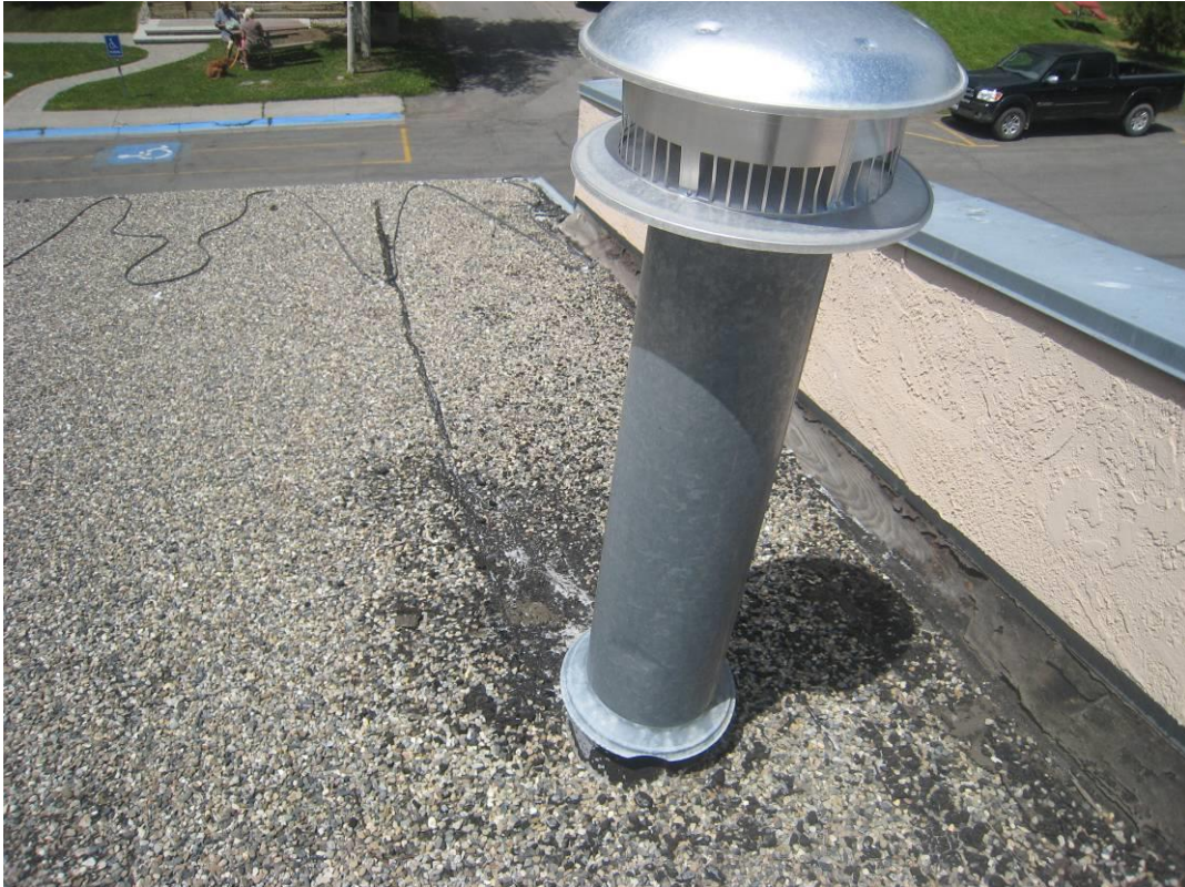
Gray material around this vent (NE corner of roof) is an asbestos containing material
