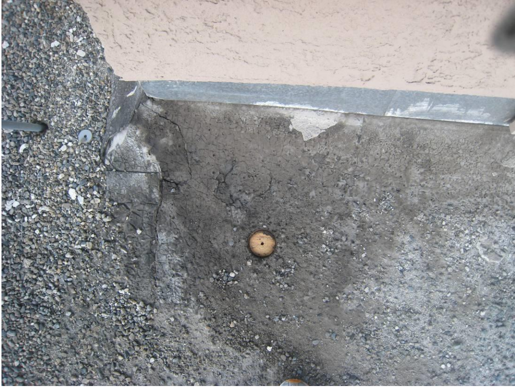
Typical roof sample; asbestos was present in felt layers.
