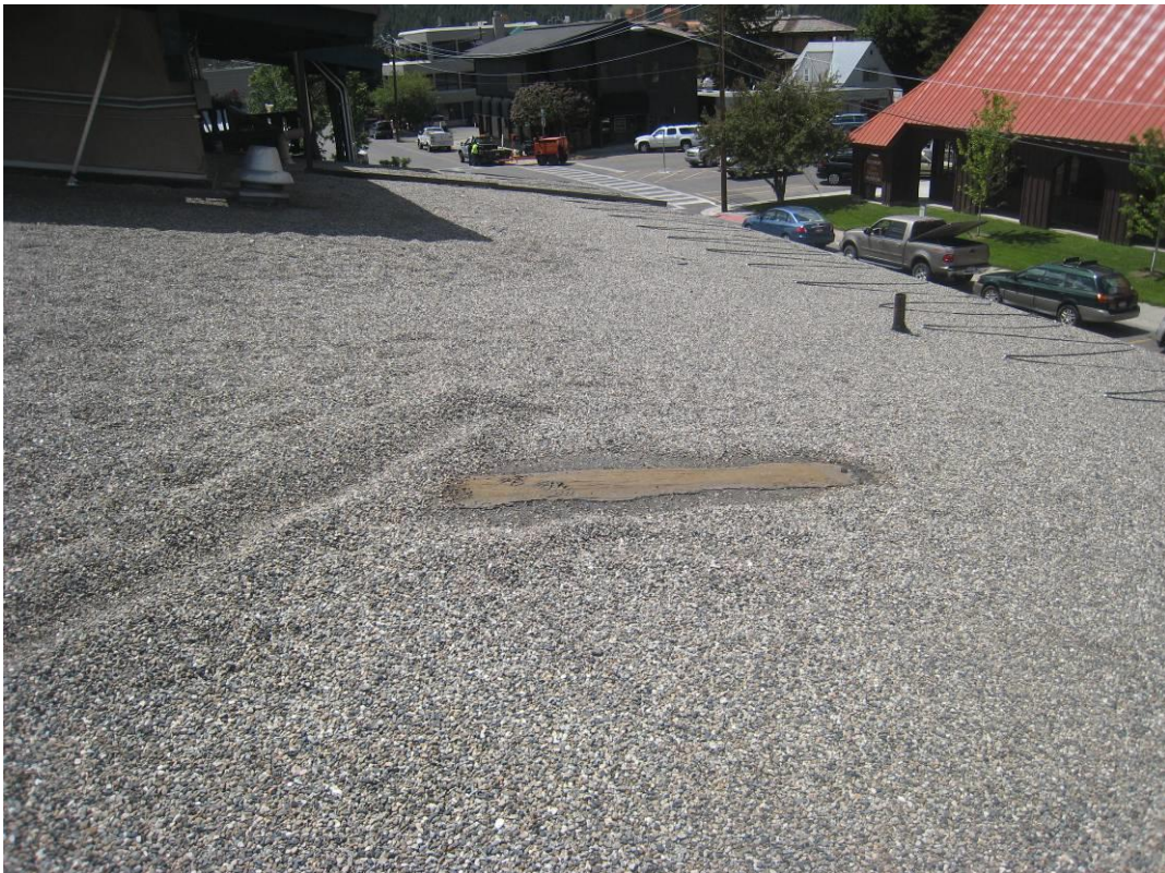
Gray mastic around the sewer pipe at the north edge of the roof is an asbestos containing material
