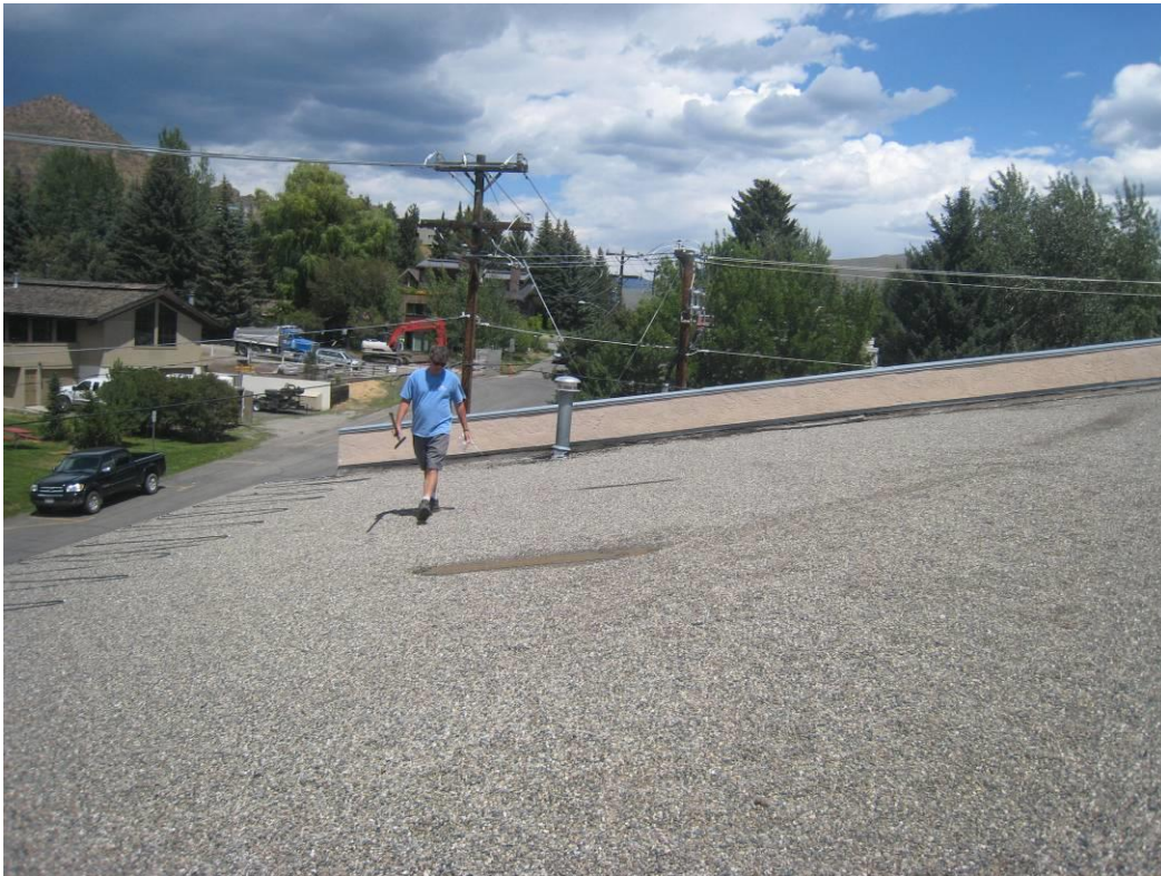
View of two patches at N side of roof; no asbestos detected in 4' x 1/2" patch (further east); asbestos was detected in 5' x 1' patch (further west).
