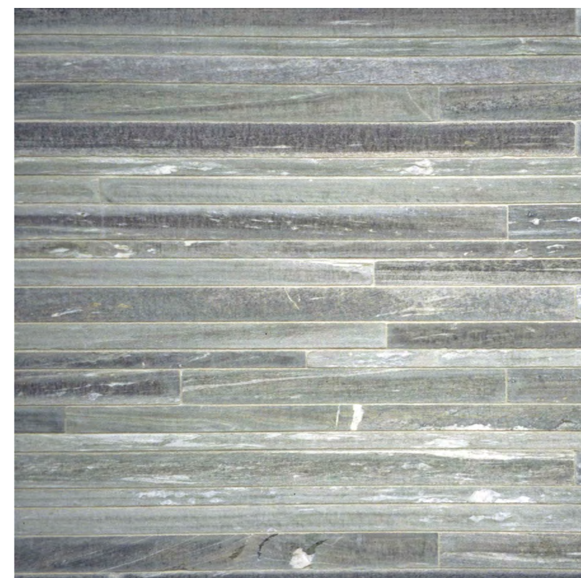
5) Stone Cladding At exterior walls
