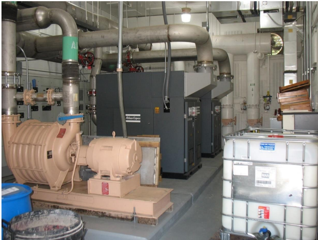
Figure 1. Existing Blower Room
