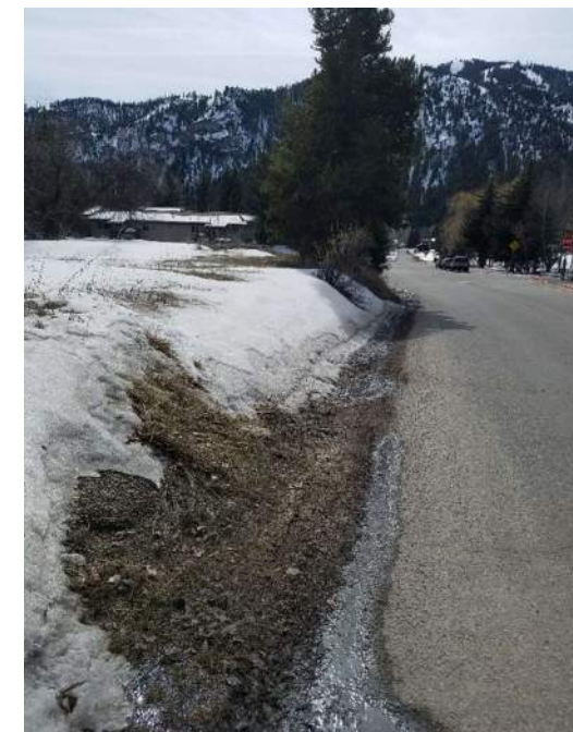
8th Street from Mid-Block Facing West- Major Grading Issues
