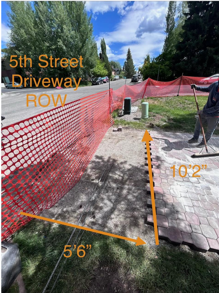
Photo with annotation provided by applicant.
