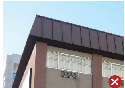
Inappropriate use of standing seam at roof.
