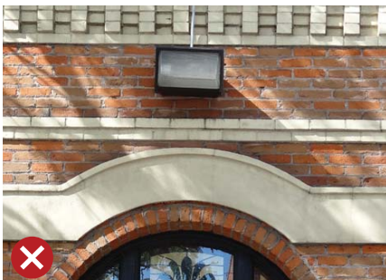
Inappropriate commercial flood light.
