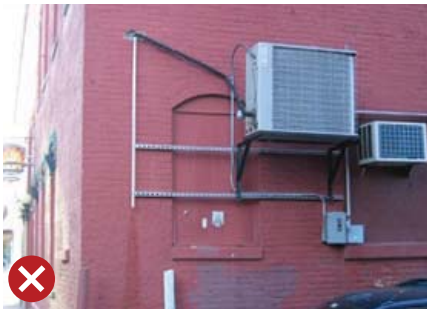
Utilities should be screened from pedestrian view.
