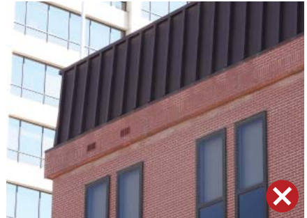
Inappropriate use of standing seam at roof.
