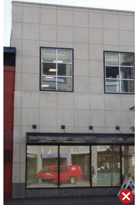
Inappropriate material selection.
