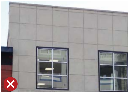
Inappropriate use of E.I.F.S. veneer.
