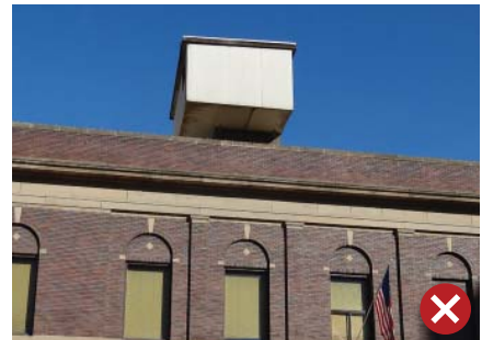
Inappropriate lack of screening for service addition.
