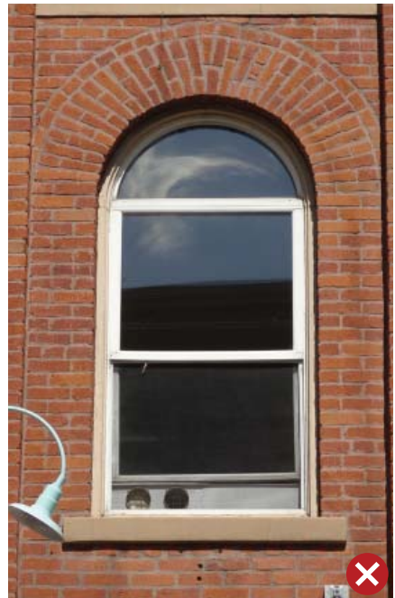
Inappropriate window replacement material.
