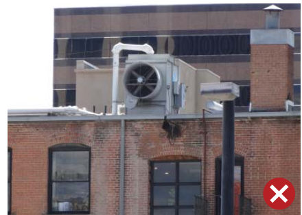
Inappropriate lack of screening for mechanical.
