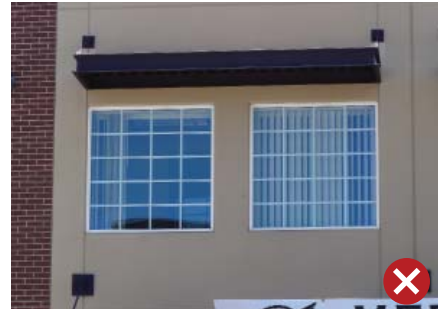
Inappropriate vinyl material.
