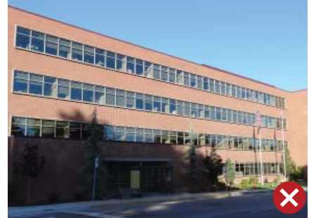
Inappropriate openings on facade.
