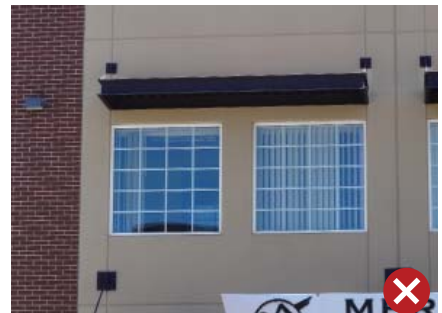
Inappropriate use of E.I.F.S. and vinyl windows.
