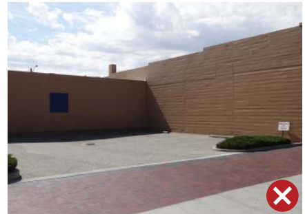
Inappropriate screening of off-street parking.
