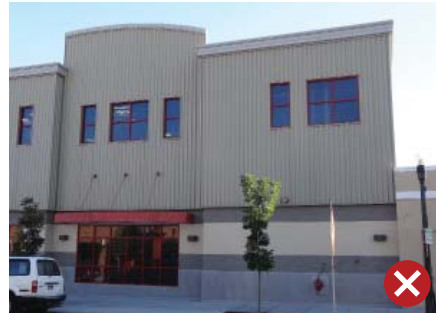
Inappropriate use of corrugated metal and CMU.
