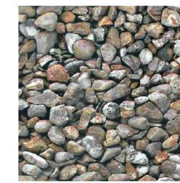
MAT 5 - Roofing - stone ballasted
