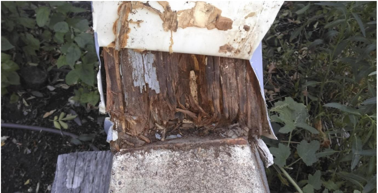
5. Existing Thrust Timber Base Rot
