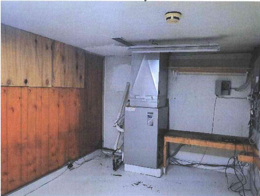
Photo 20: Gas furnace in furnace room Note: strong diesel (heating oil) odor; concrete floor
