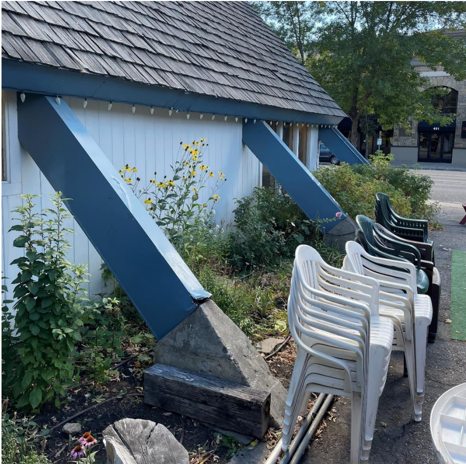
4. Typical Thrust with Typical Rot as Reviewed
