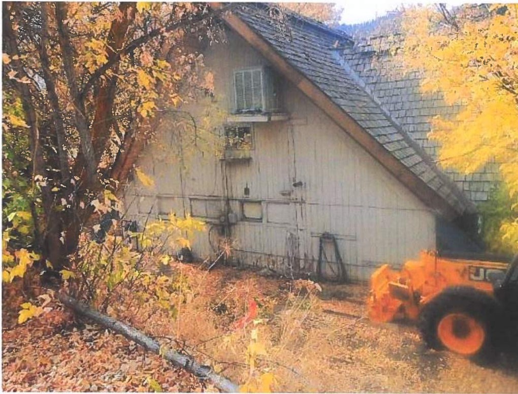
Photo 7: Looking S toward rear of subject building Note: property corner marker between Lots 3 and 4; forklift
