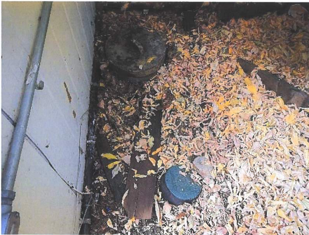
Photo 9: access conduits observed outside rear corner of building Note: appear to be water related
