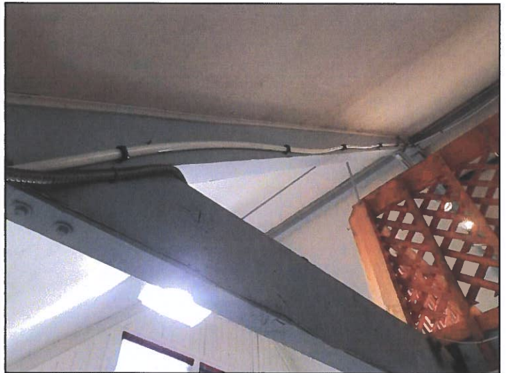
Water line is routed through visible interior space.
