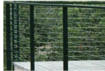
GUARDRAIL 1 (GR-1): BLACK STEEL CABLE RAIL
