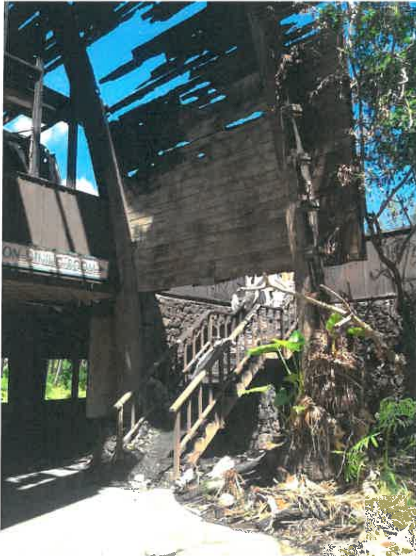
Coco Palms has high integrity but is in bad condition (Photo Courtesy Jessica Puff, SHPD)
