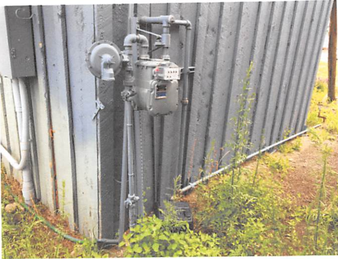
Existing Gas Meter
