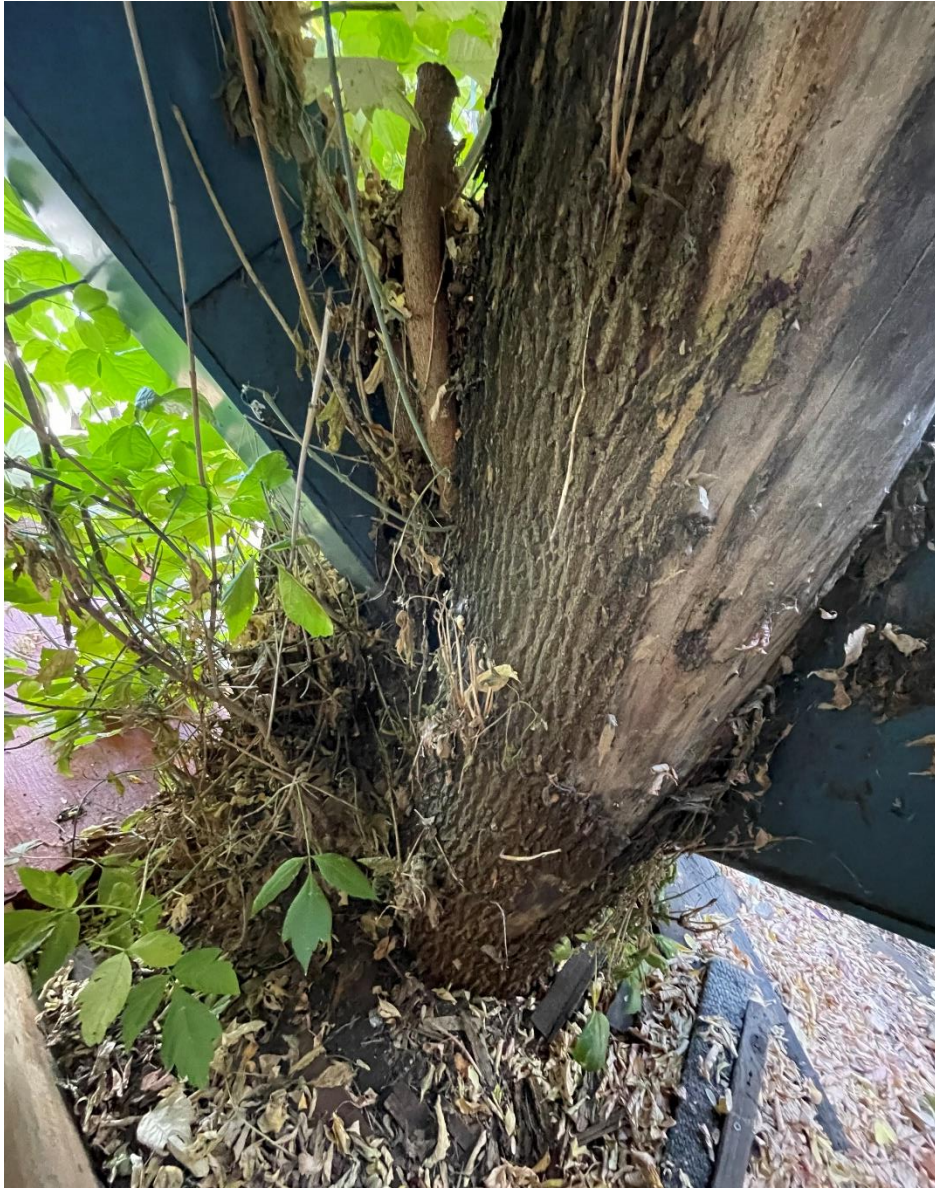
6. Tree Growth Compromising Foundation
