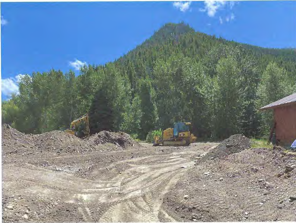
Site improvements consisting of excavation of unsuitable soils and placement of structural fill was concentrated on the west side of the project site where restaurant and ponds were removed. 1Jul20
