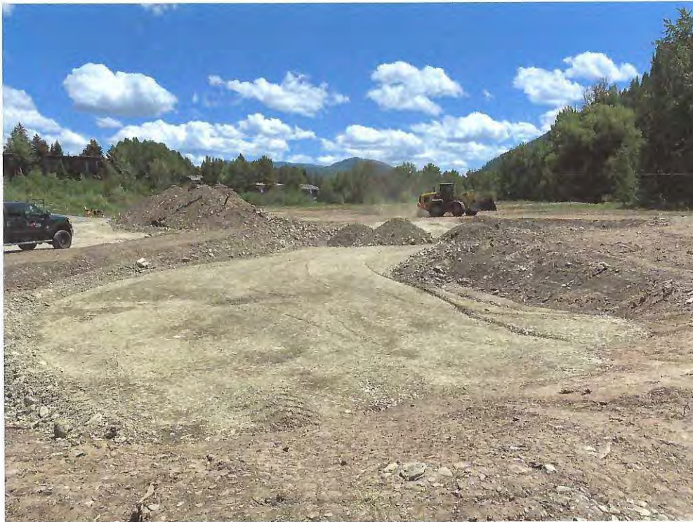
Up to 5 feet of imported sand and gravel placed to match adjacent existing grade. 1Jul20
