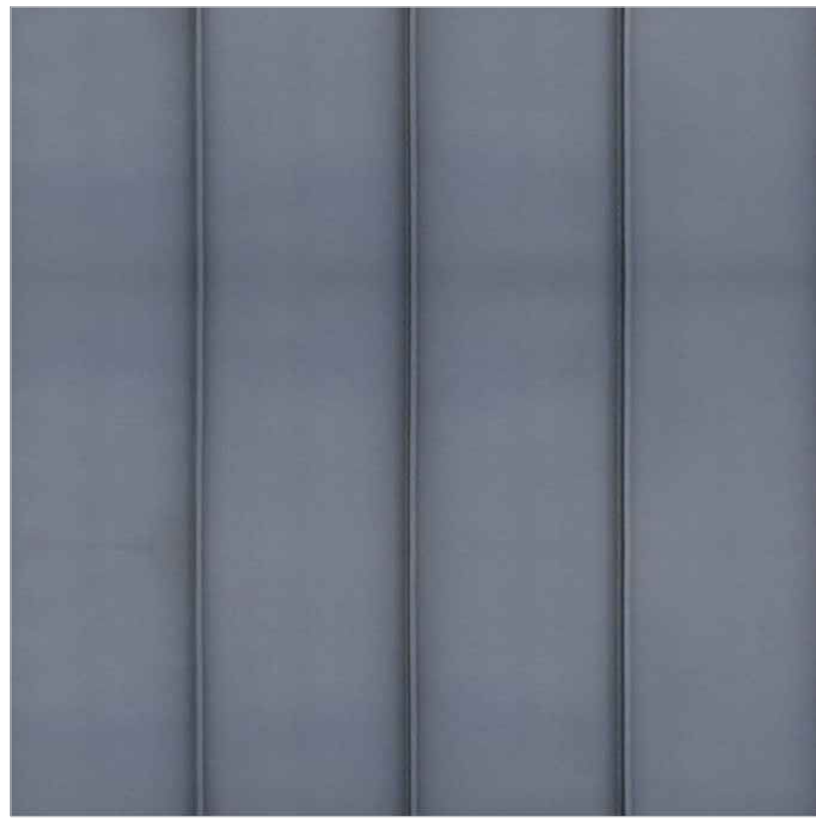
6) Zinc At chimneys & parapet caps
