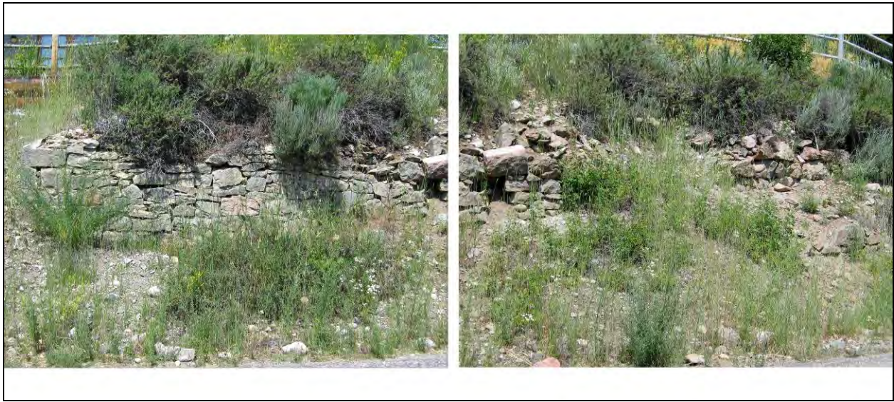
Figure 17a. View of east facing wall along Exhibition Boulevard looking west. Digital Image WS 37 # 20.
