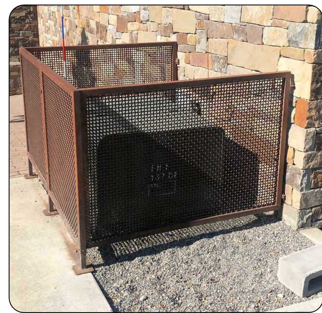
PHOTO: TRANSFORMER COVER EXAMPLE
