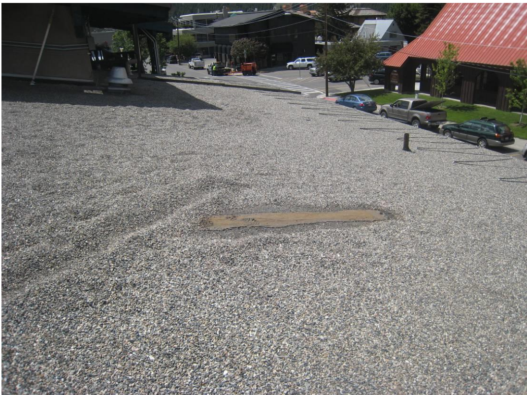
Gray mastic around the sewer pipe at the north edge of the roof is an asbestos containing material
