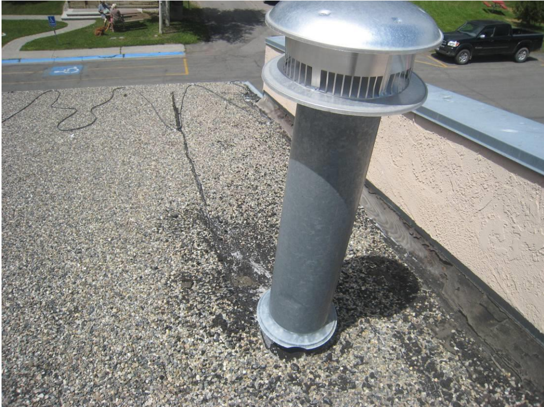
Gray material around this vent (NE corner of roof) is an asbestos containing material
